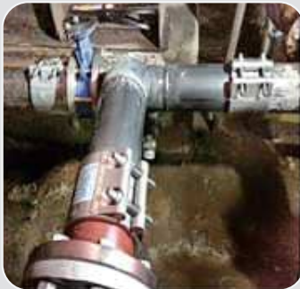
▶ Water treatment works
