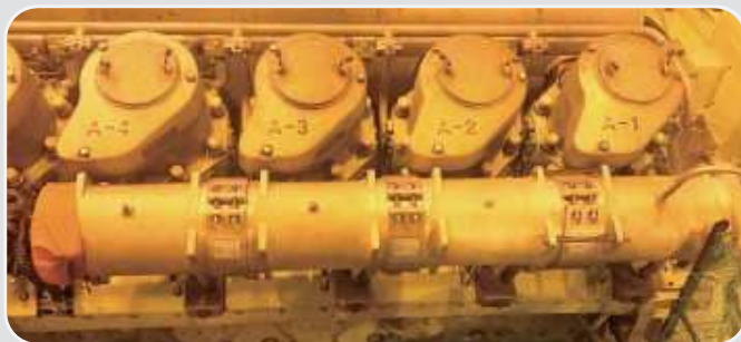
▶ Nuclear plant emergency generator suction pipe
