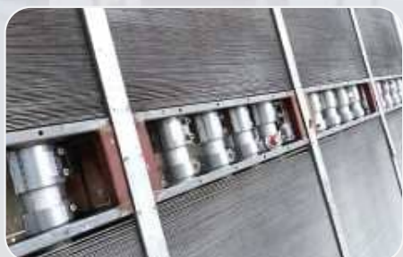
► Installation on an incinerator cooling water line.
