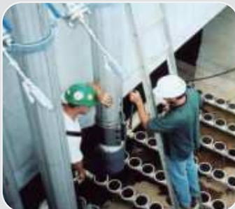
▶ Water treatment plant
