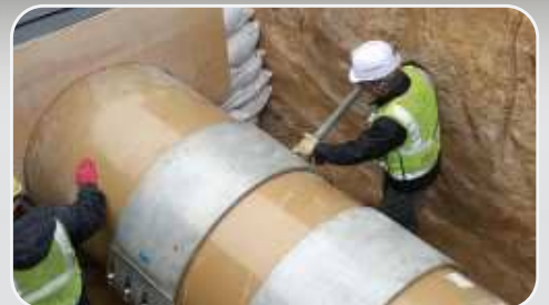
▶ GRP piping connection
