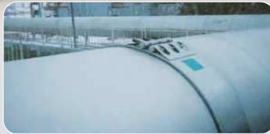
▶ Canadian power plant cooling line
