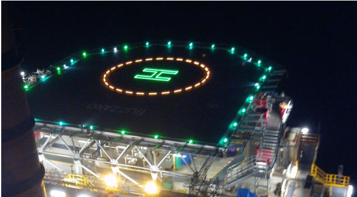
Figure 2 - Helideck Lighting System
