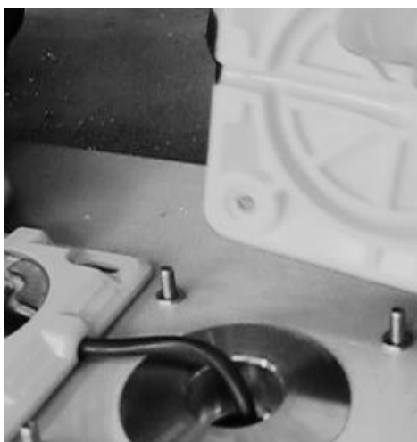
Figure 22 - Installed Cable Bushing
