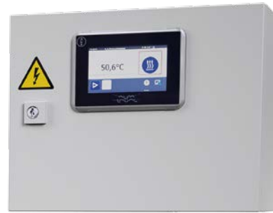
EHS-71 control unit.
